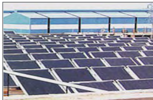
Fig 3.15: Solar Panels to trap solar energy
